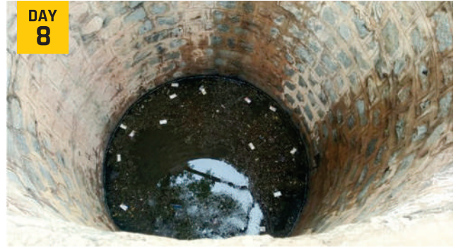
Cleaning of open well by VIOM employees at Danapura Village (25th Nov 2021)
